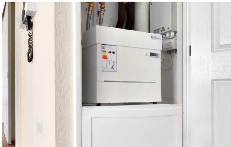
Figure 3 A photo showing a GSHP installed at a property.
